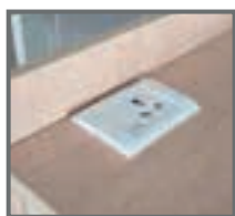
In built Sockets
